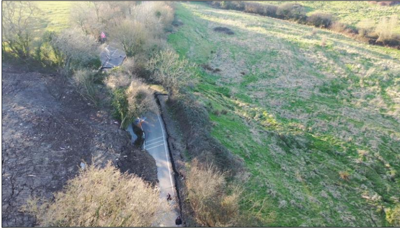
The extensive landslip at Lyneham Banks has caused enormous problems in the area when a large section of the B4069 disappeared completely
