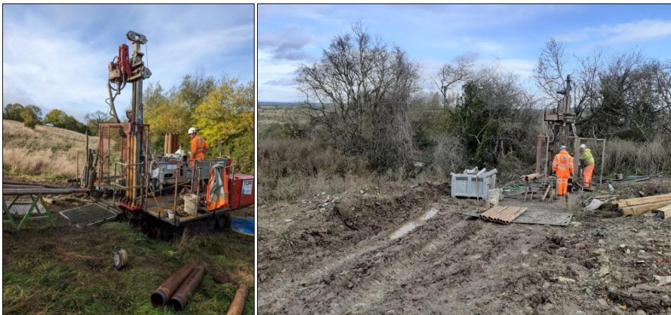
A detailed ground investigation with boreholes was undertaken to help design the remedial measures
